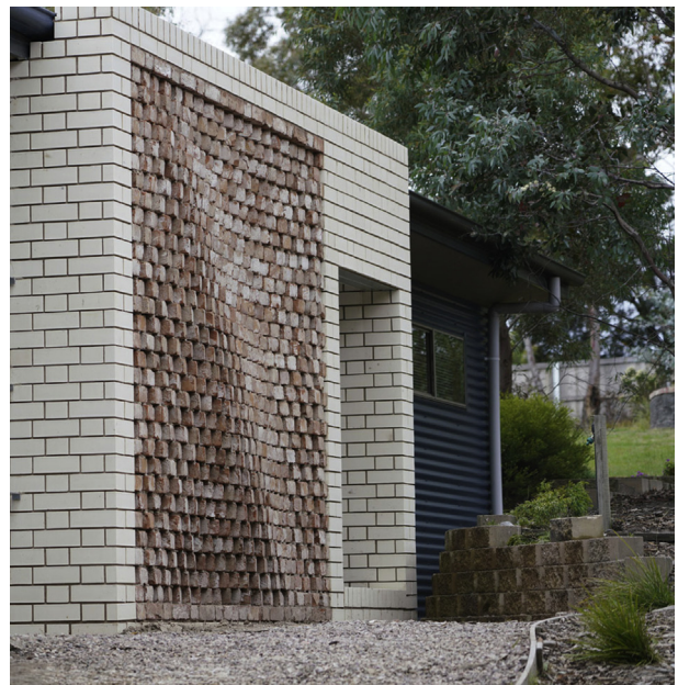
Fig. 9 Fologram’s complex curved wall at UTAS, an early example of AR guided bricklaying, © Fologram ( https://www.archdaily.com/908618/this-is-how-a-complex-brick-wall-is-built-using-augmented-reality ).
