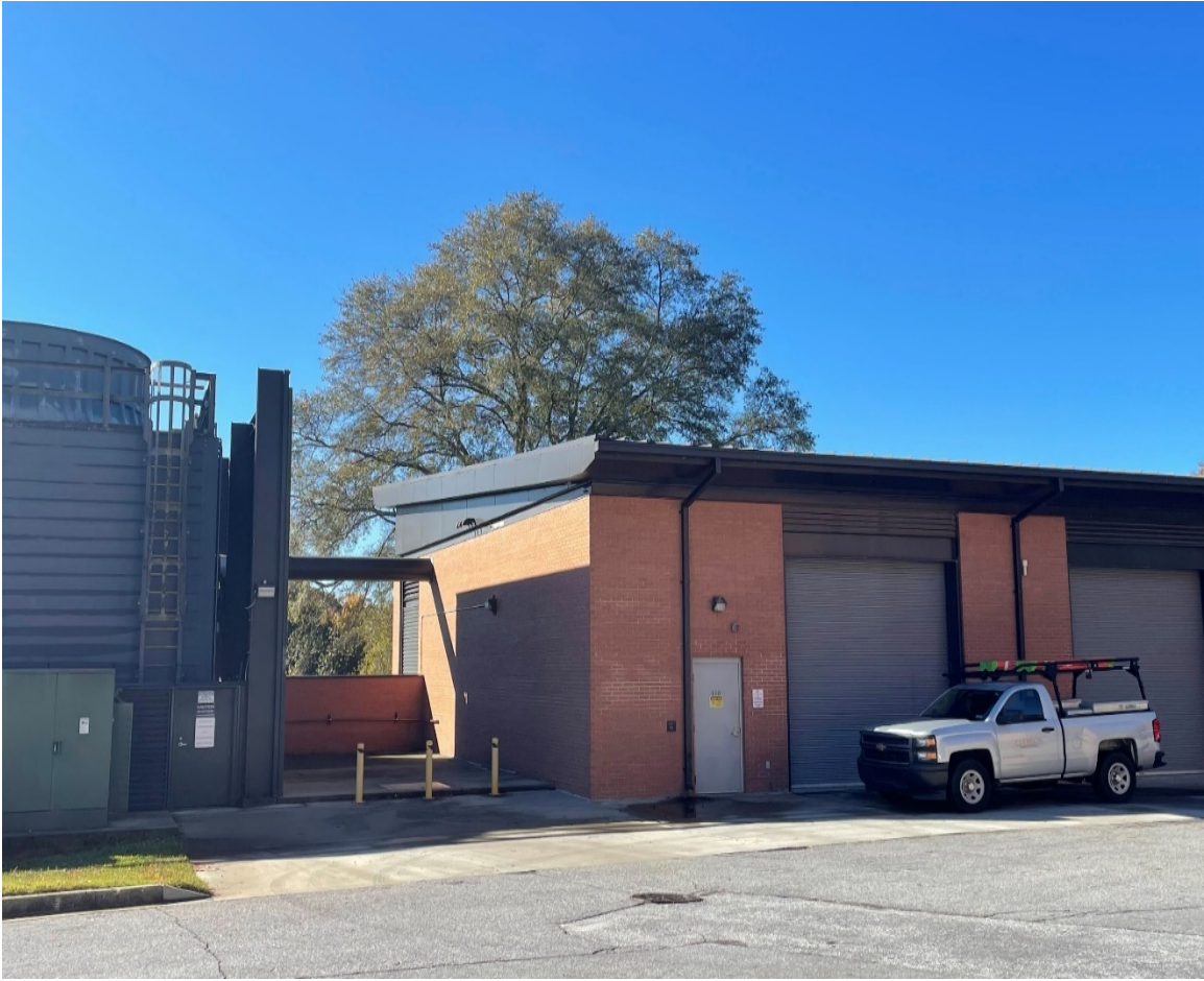
Figure 1.4: Chiller plant behind Fluor Daniel Engineering Innovation Building connected to cooling towers at Clemson University
