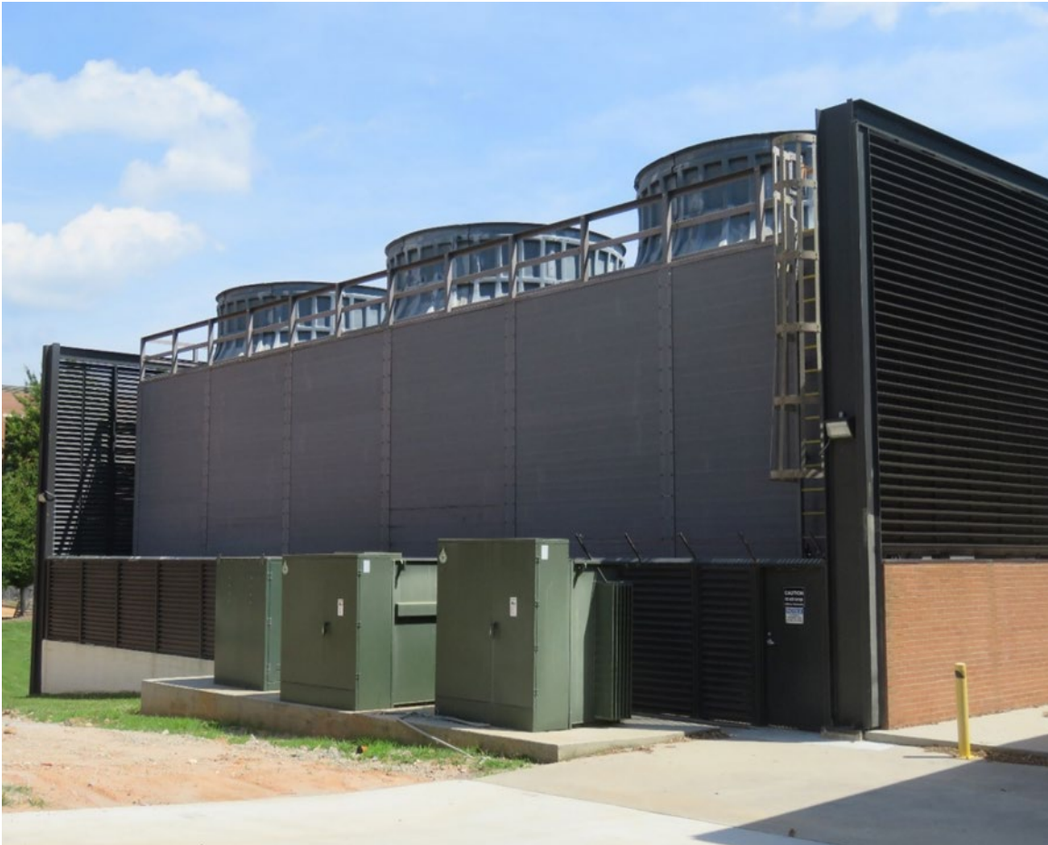
Figure 1.3: Cooling towers behind Fluor Daniel Engineering Innovation Building at Clemson University
