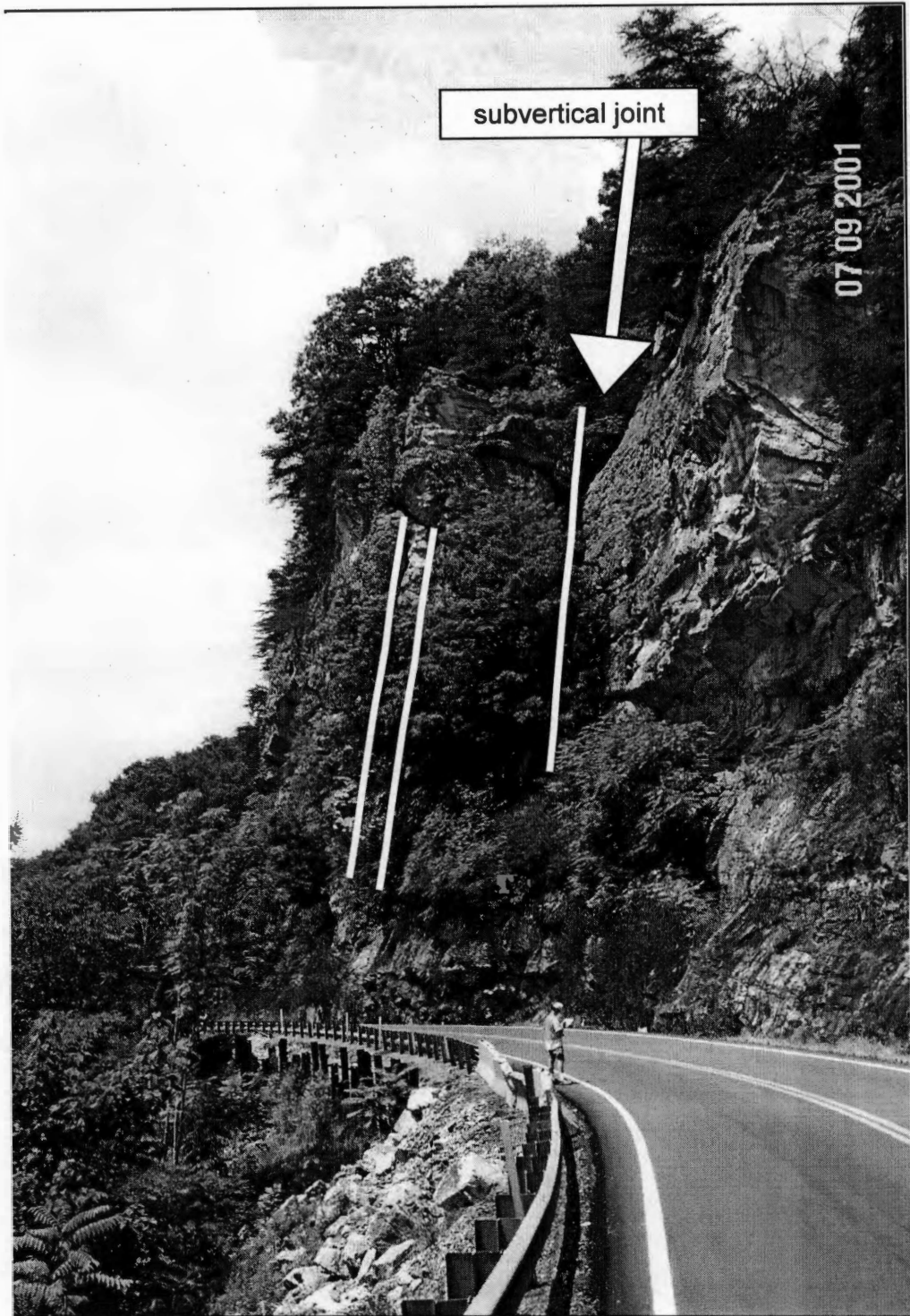
FIGURE 4. Roadcut B4 on Tennessee SR 30 showing large rock mass separating from slope face primarily along particular subvertical joint (arrow). View is to south.
