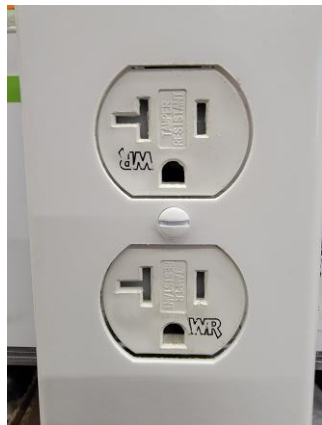
Figure 9: NEMA 5-20 wall outlet. (Own photo, 2021)
