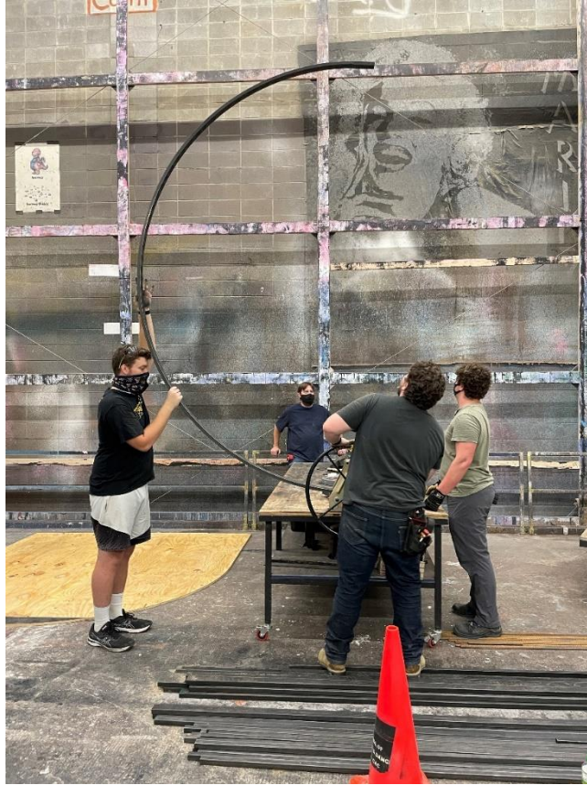
Figure 72: Technical Director, Mr. Christopher Sheriff works with work-study students to manipulate box steel to match the outline of the bridge balcony platform
