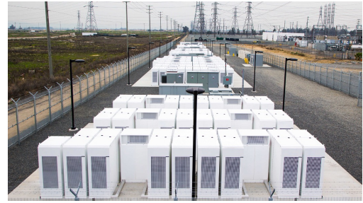
(b) Batteries used to storage energy for electric power grids.
