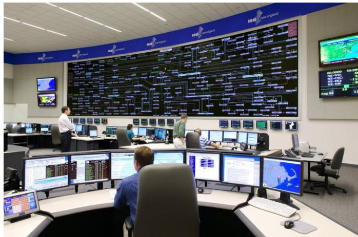
Figure 1. ISO New England Power Grid Monitoring Room [15]
