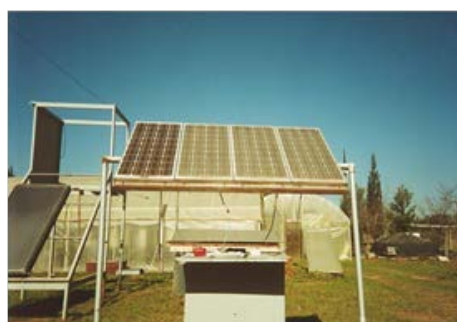
Figure 2. Four solar panels.
