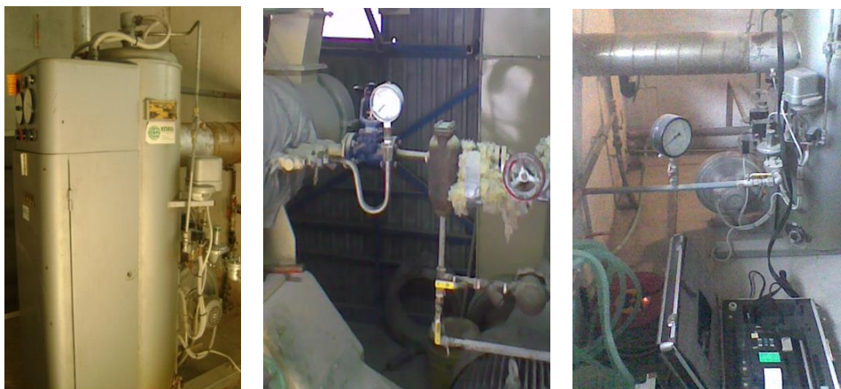
Figure 2: Installation of sensors and measuring devices at the critical points of the combined feed production technology flow
