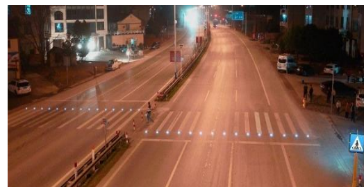
Figure 19. Using pedestrian lighting system, source: ( https://www.ellumin.com/project/non-light-control-area-intelligent-pedestrian-system%EF%BC%88urban-type%EF%BC%89/ )
