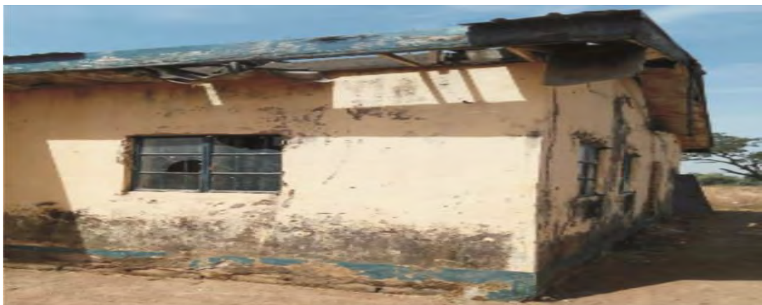
Figure 4.20: Abandoned Primary Healthcare Centre in one of the Local Government Source: Fieldwork, 2018.
