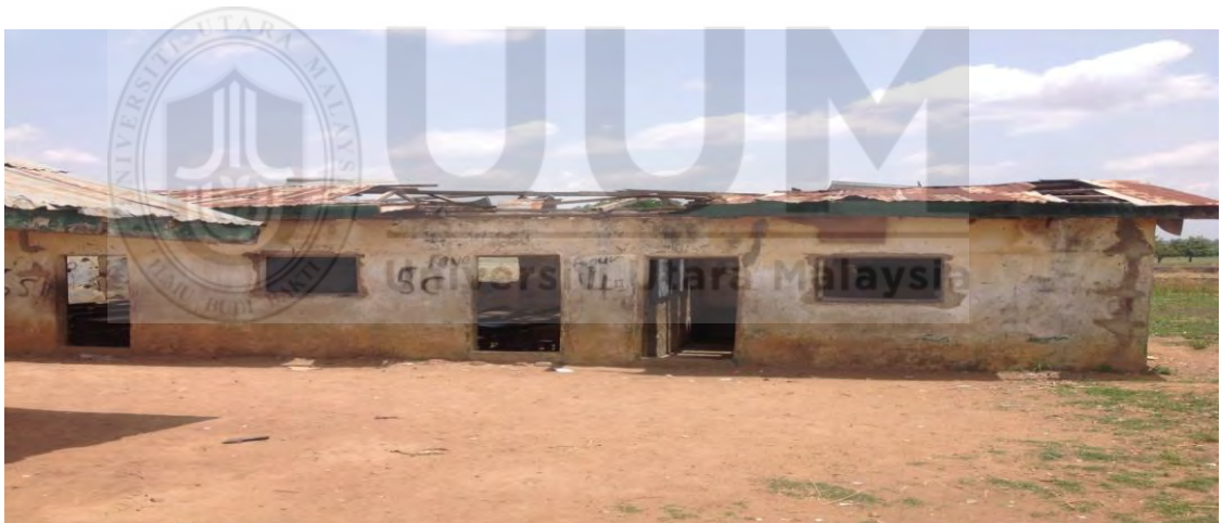
Figure 4.18: Abandoned Primary School in one of the Local Government Areas Source: Field work, 2018.
