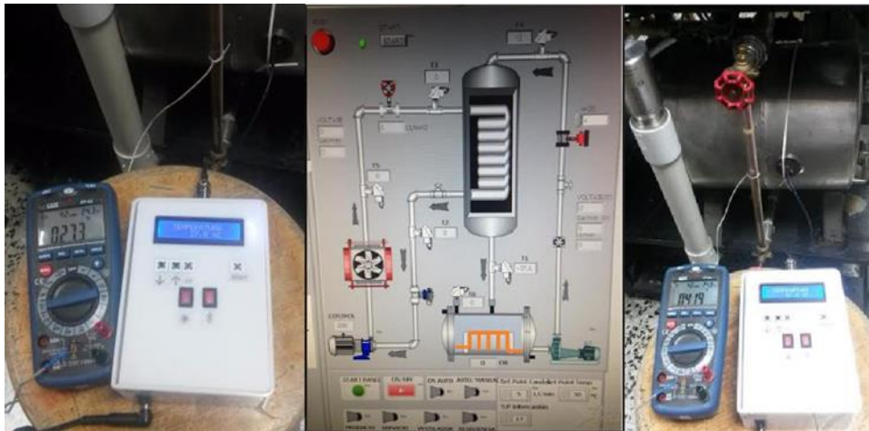
Figure 21. Measurements in the thermal plant.
