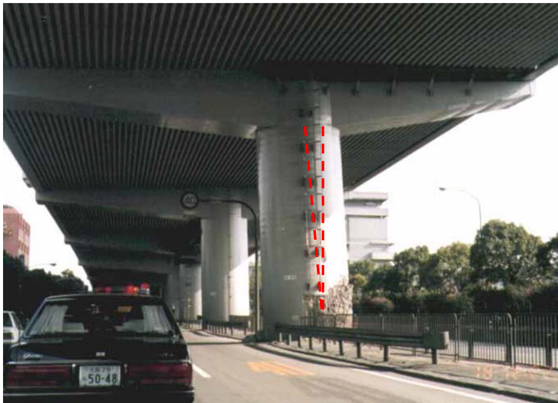
Figure 1.4 Residual drift of bridge columns from Kobe, Japan earthquake
