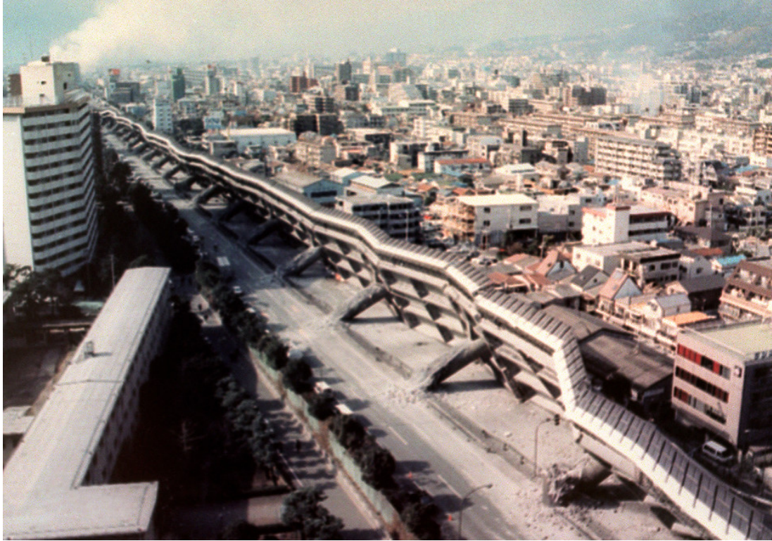
Figure 1.3 Bridge collapse from Kobe, Japan earthquake
