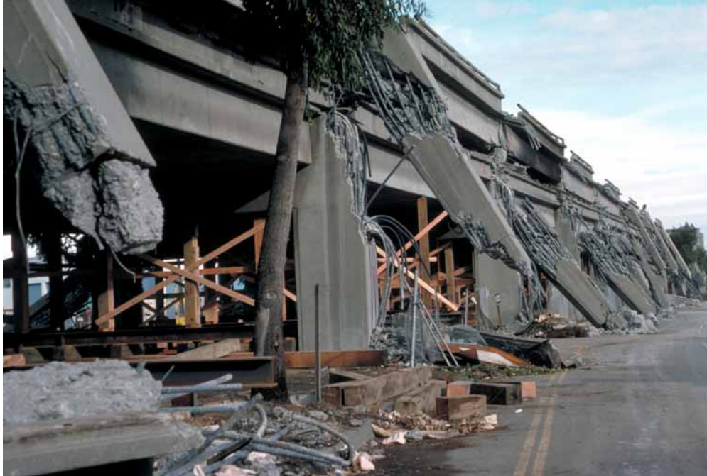
Figure 1.1 Bridge collapse from Loma Prieta, CA earthquake
