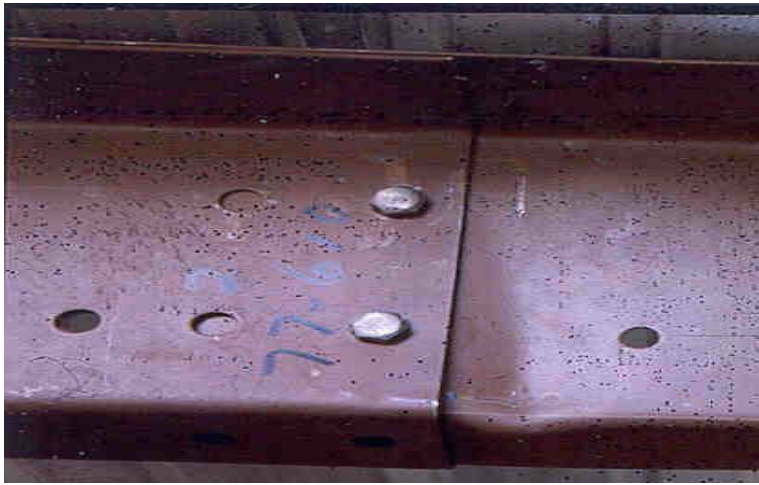
Figure 3.1.1 Photograph of Failed Purlin at End of Lap
