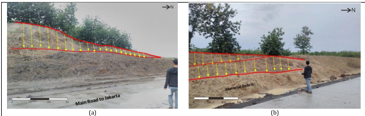
Fig. 1. Slope failure along the: (a) STA 438+000; and (b) 439+000 segments at end of the construction stage
