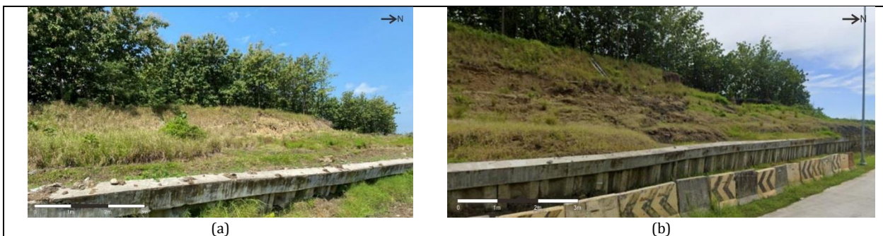
Fig 2. Slope failure along the STA 438+000 segment during: (a) early road operations; and (b) a recent failure in 2021
