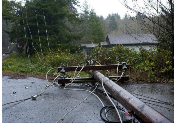
Figure 15. Fallen Power Lines - Library Sample Image [33]
