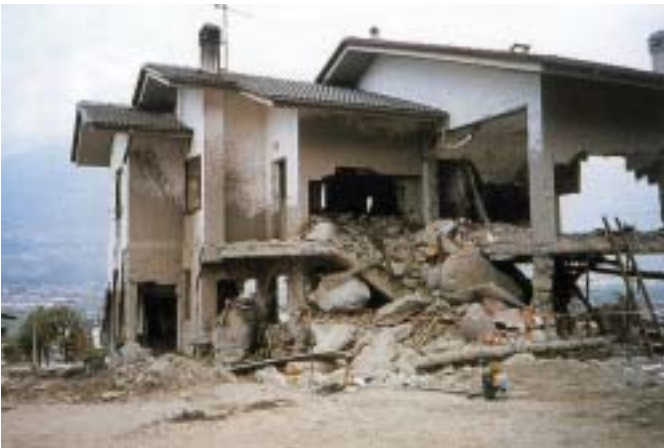
Photo 4 Pollein – Effects of debris flow (author: local media).
