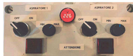
Fig. 5. The control panel with the voltmeter of the mains voltage, two rotary switches to turn on/off the aspirators, the potentiometers to set the speed, and two voltmeters/ammeters indicating the voltage and current supplied to the aspirators.
