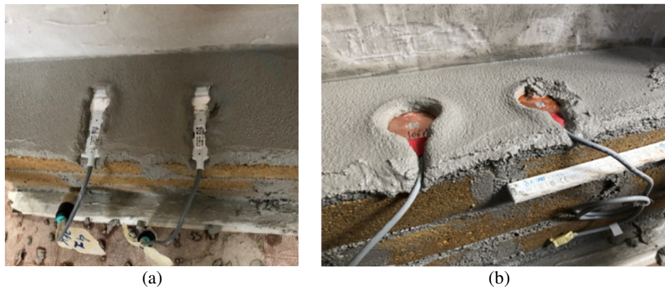
Figure 3. Installation of the sensors in the mortar bed-joints: (a) ceramic sensors; (b) capacitive sensors.
