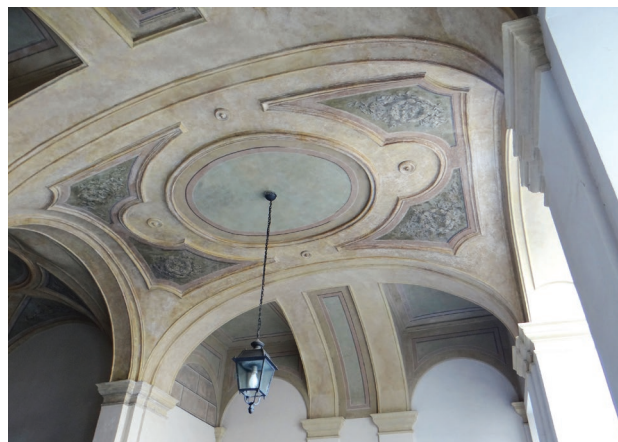
Figure 1. The main banded vault of the atrium of Capris di Cigliè Palace (photo by M. Vitali).
