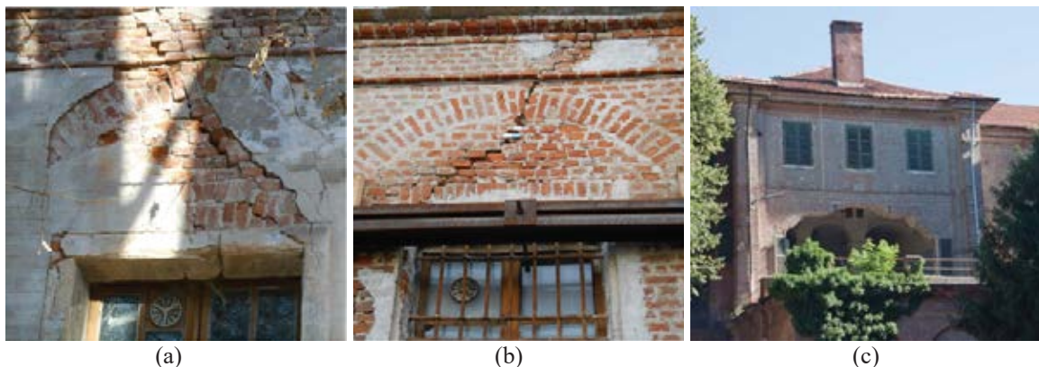
Figure 1: (a-b) some cracks on the various facade of the building (2015); (c) collapse of a portion of the southern façade (2016).
