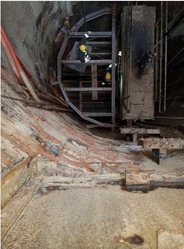
Fig. 7 Installation of the first support structure in the shaft of the Carbosulcis mine, Seruci site.
