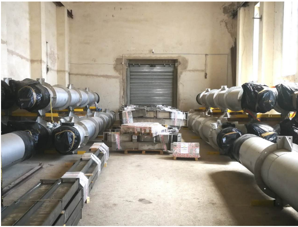
Fig. 2 The central modules of the column stored at Carbosulcis S.p.A., Nuraxi-Figus site, ready for installation.
