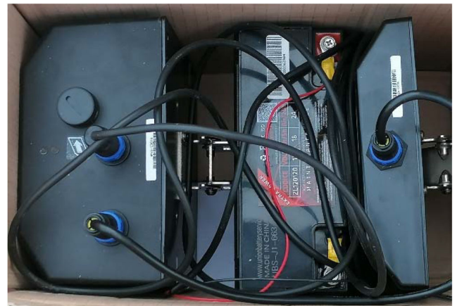
Fig. 1 Photo of BT and WF scanners used during the on-field tests composed by the scanner, the battery and the antenna
