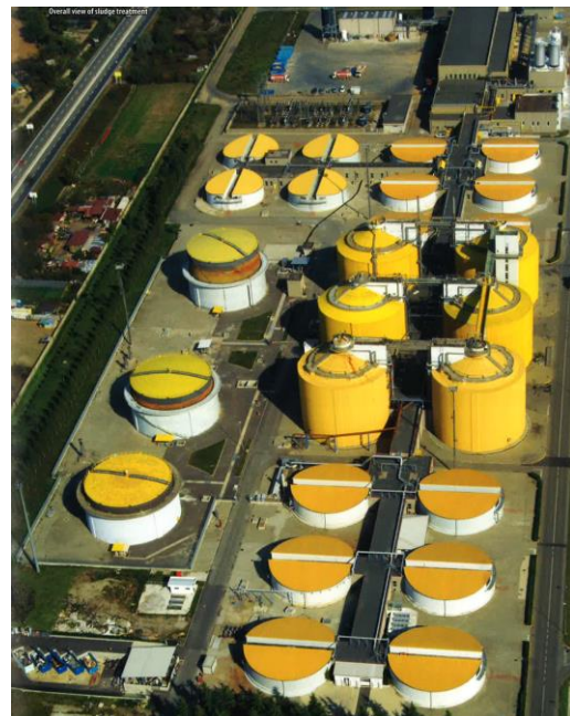
Figure 2: Photo of the sludge treatment line.
