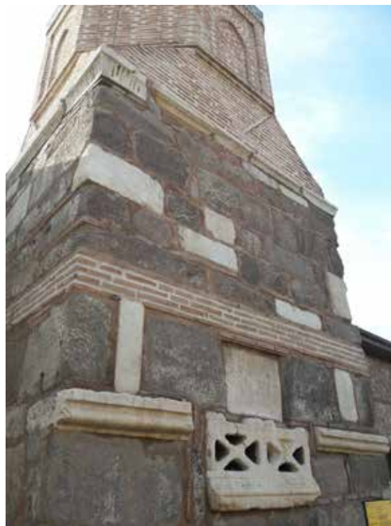
Roman ancient parts inside the construction of the minaret of the recent mosque near the citadel area.
