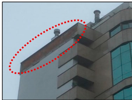
Figure 1. View of the region with detachment of stone elements (façade facing southeast)
