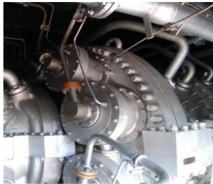
Gambar 13. Annular Combustion Chamber PLTGU Keramasan
