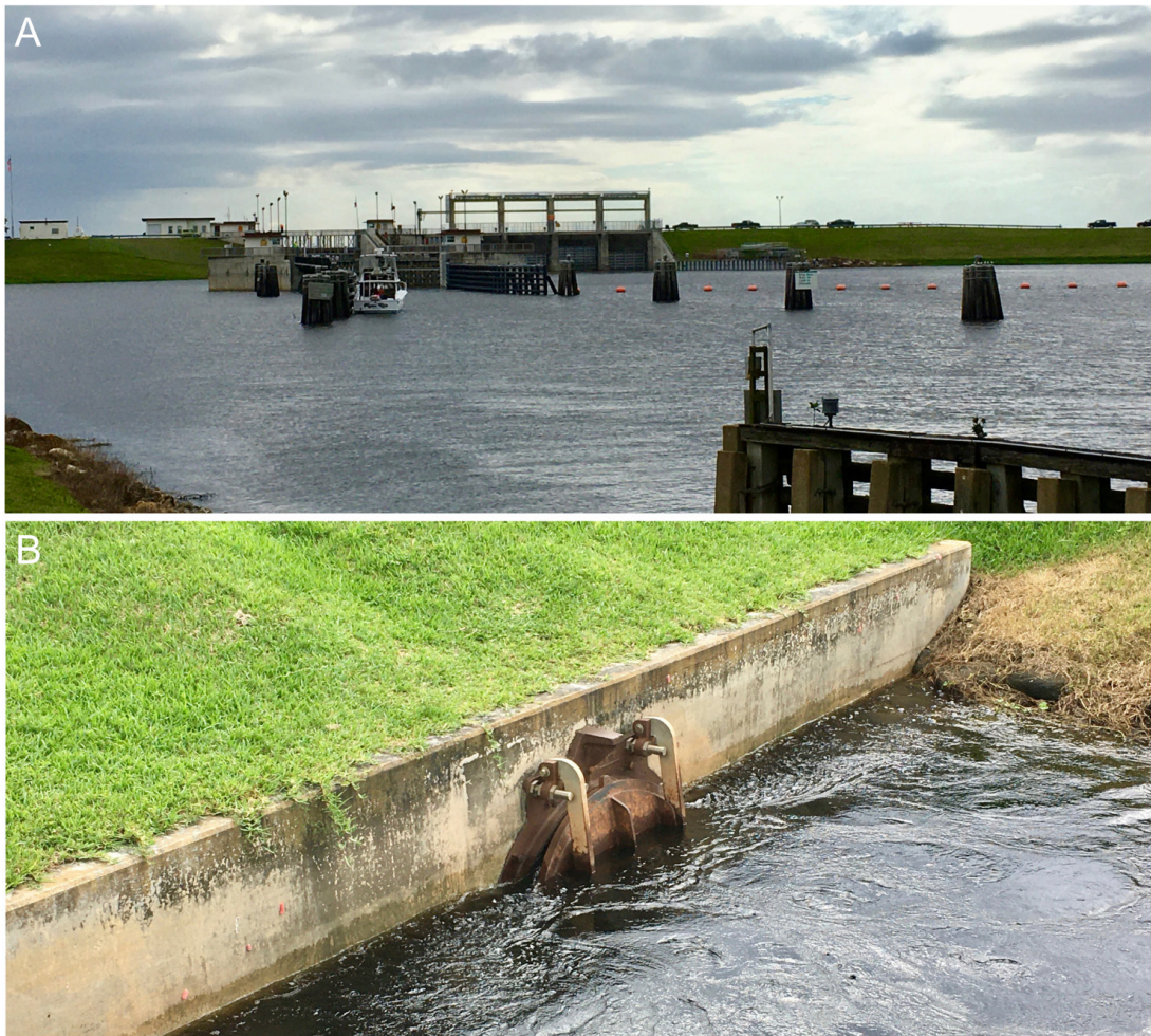
Fig. 5- The lock system at the St. Lucie connection to Lake Okeechobee: A) the lock as viewed from the St. Lucie Canal that raises or lowers boats from the elevation of Lake Okeechobee, B) an outlet for water discharged from the lock to lower the water level within the lock.
