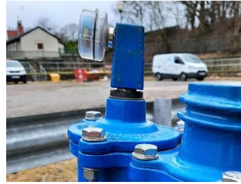
Figure 2.2 A FIDO Bug attached magnetically to a hydrant
