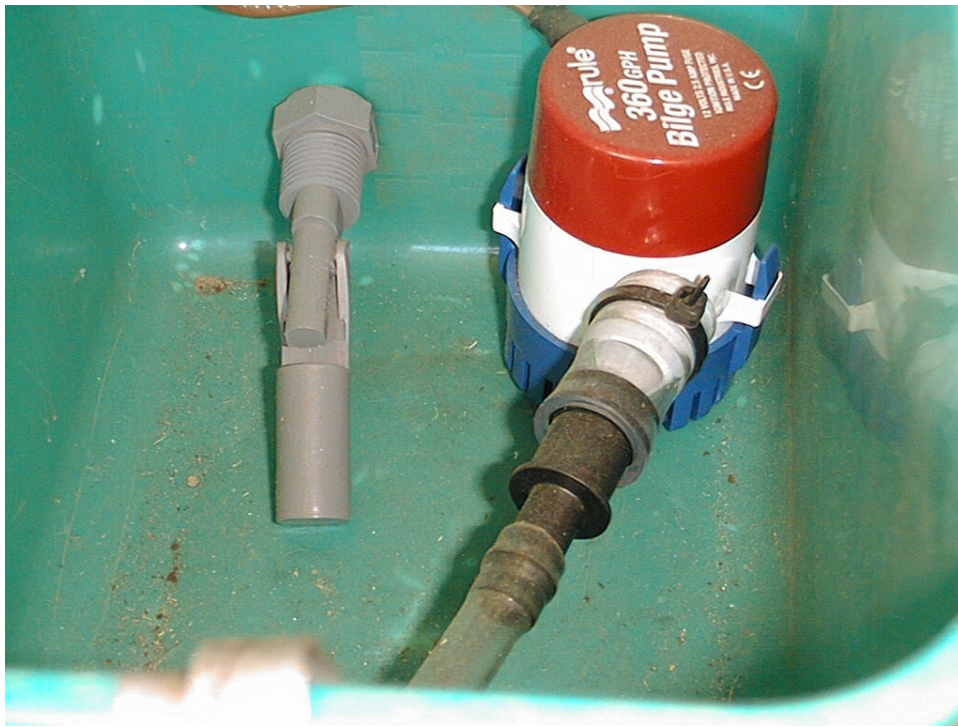
Fig II.4 Bilge pump and level switch mechanism for pumping treated effluent out
