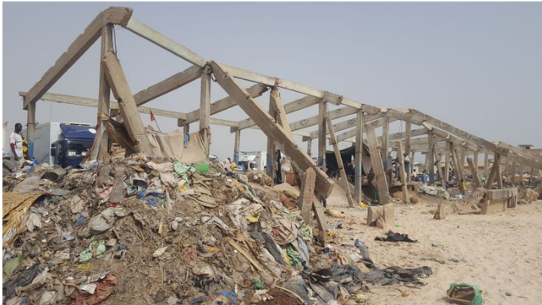
Figure 1. Destruction of building that used to house pirogues (wooden fishing boats), Guet Ndar
