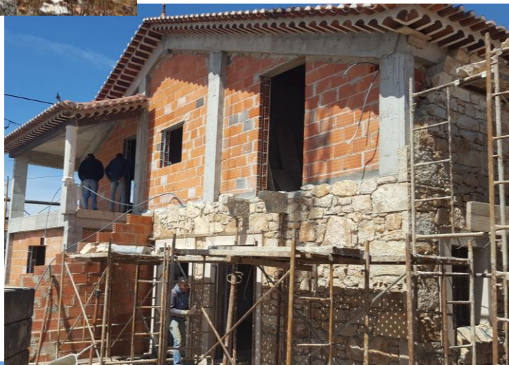
Picture 17 - House Maria do Bento during the restorations in Serra de Santo António
