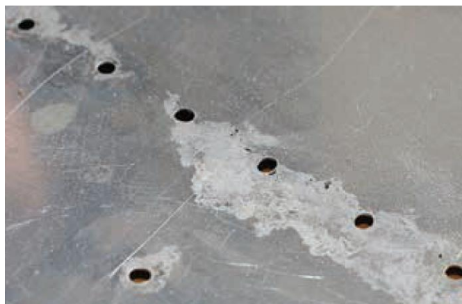
Figure 2.4: Example of general or uniform corrosion [3].
