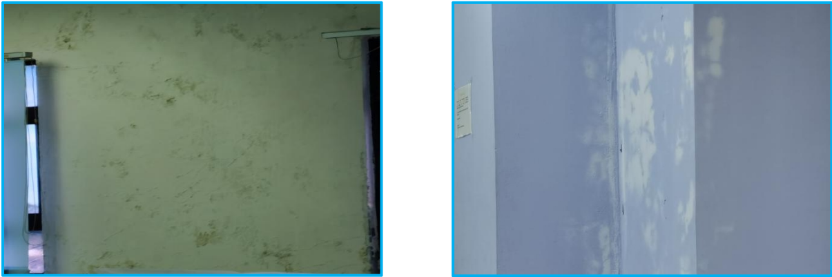
Figure 4.19: Minor defect of interior wall painting finishes
