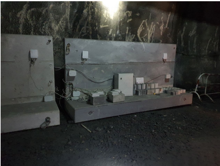
Figure 6.2: Corrosion and structural health monitoring of tunnel precast concrete segments for mining tunnel demonstrator in EnDurCrete Project
