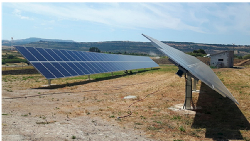
Figure 3. Stand-alone PVIS installed in Uri (Sassari, Italy).
