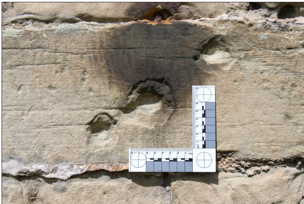
Figure 9: Photograph of scars showing prominent outer spalling at Ashby Castle, Leicestershire
