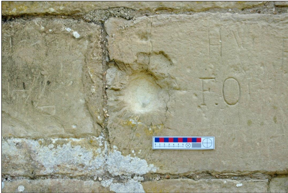
Figure 2: Photograph of a suspected artillery impact scar at Old Wardour Castle, Wiltshire
