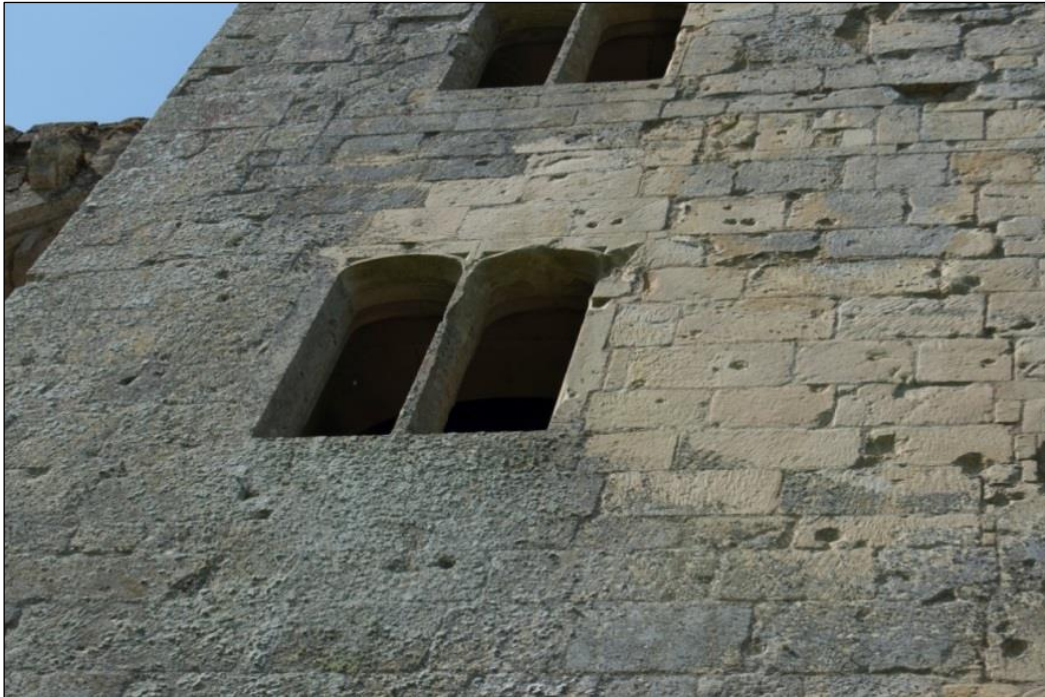
Figure 35: Photograph of a window opening on the 'right' tower of the Old Wardour gatehouse, illustrating the visual contrast for identifying scars on the bare ashlar, and on surfaces covered in textured lichen
