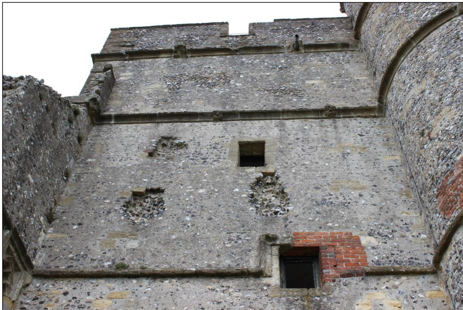
Figure 13: Photograph of artillery damage at Donnington Castle, Berkshire
