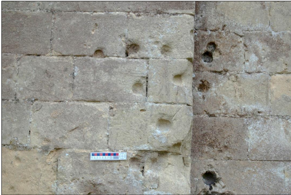
Figure 16: Photograph of possible hail shot impacts on St. John's church, Devizes, Wiltshire
