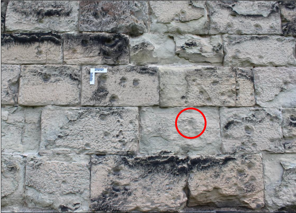
Figure 41: Photograph of impact scars at Ashby Castle. Circled is a scar where the original surface level has been lost due to weathering
