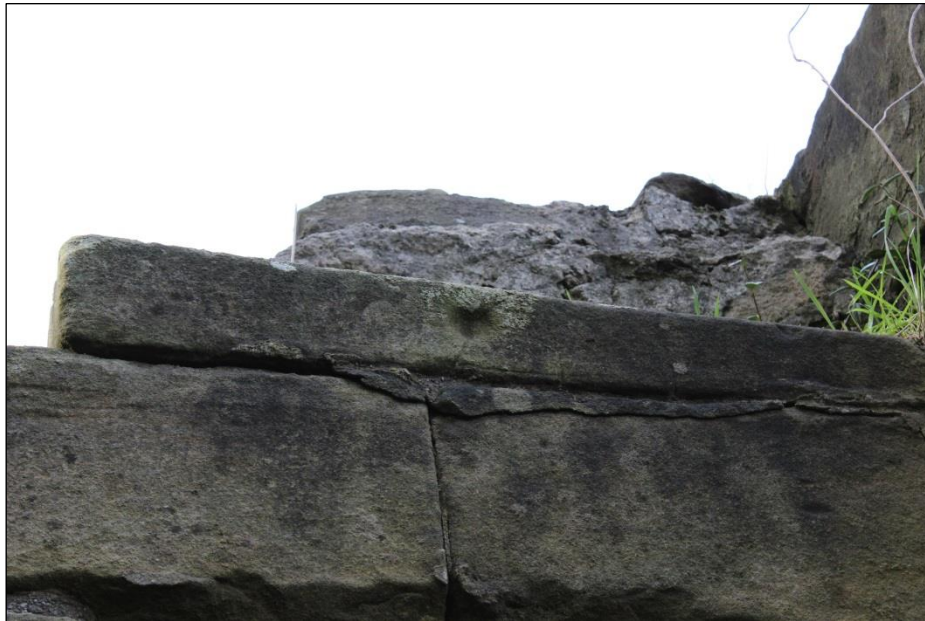
Figure 3: Photograph of an impact scar on a surviving castle wall section at Pontefract Castle, West Yorkshire
