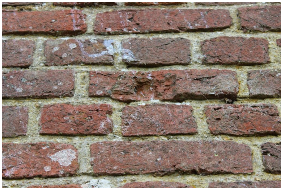
Figure 12: Photography of an impact scar on a brick wall at Basing House, Wiltshire
