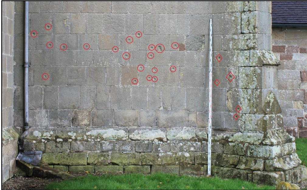
Figure 83: Grouping of scars on eastern end of the south aisle exterior wall bearing measured scars C01-26. Scars are indicated by red circles for clarity, red diamonds indicate scars C01-05 on the angled buttress. This wall faces towards Moreton Corbet Castle
