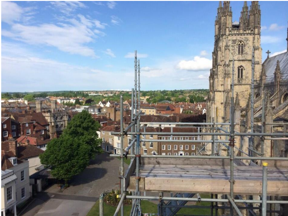
Figure 12. Canterbury Cathedral is having an extensive programme of conservation works to the Northern Towers, the Nave, and Trinity Chapel © Christopher Moore
