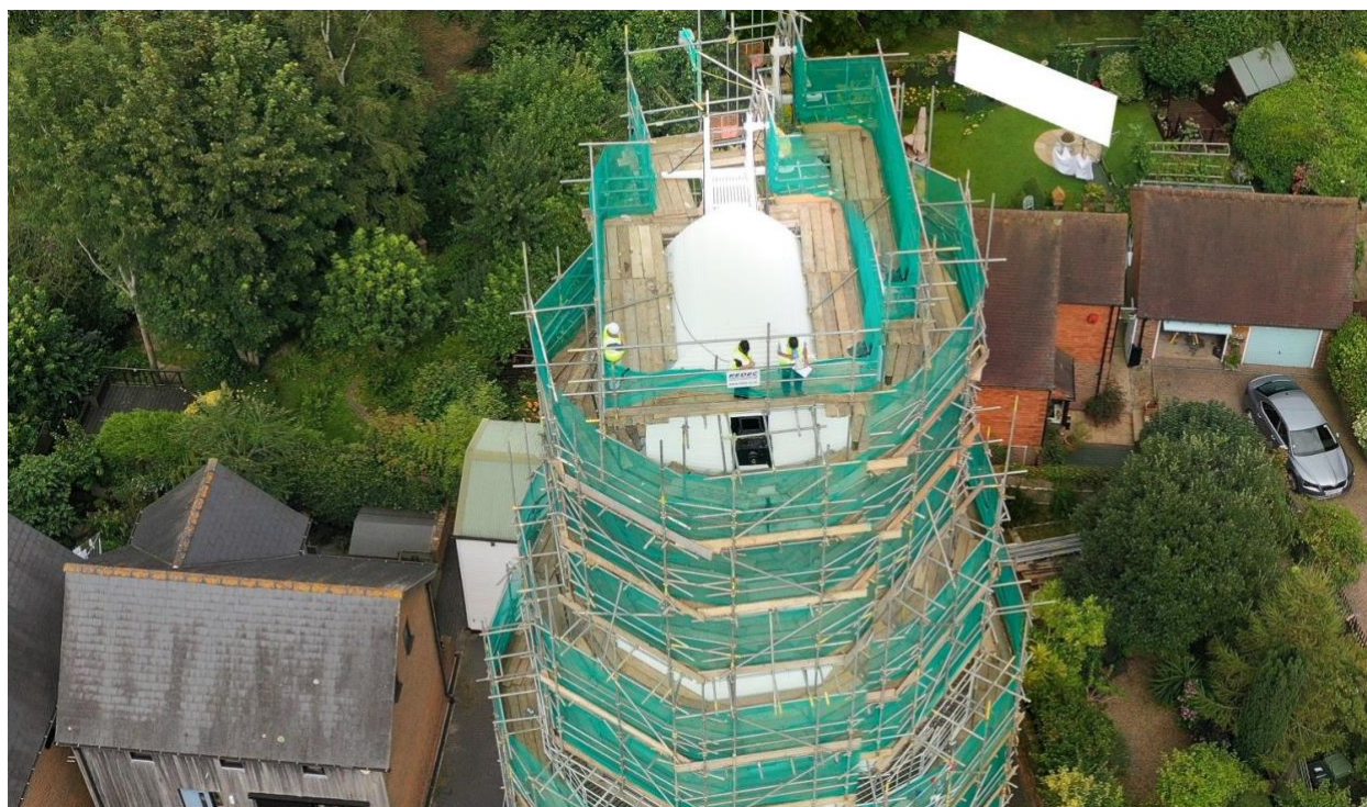
Figure 13. The KCC owned and operated Union Windmill in Cranbrook (one of the tallest mills in the UK) received a significant programme of restoration work between 2021 and 2022 © Nick Vinall / Hawkeye Media
