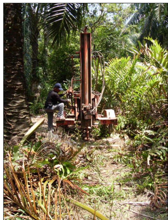
Figure 4. Core drilling process through hydraulic drive rotation method using flight-mounted solid auger applied in Sungai Batu Archaeological Complex
