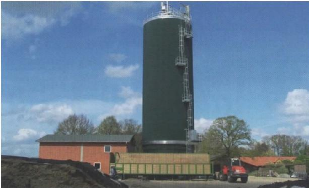
Figure 11.7. BGP 49, in front the feeder for solids, behind the vertical digester, besides the operations and farm buildings (Source: FNR 2009).
