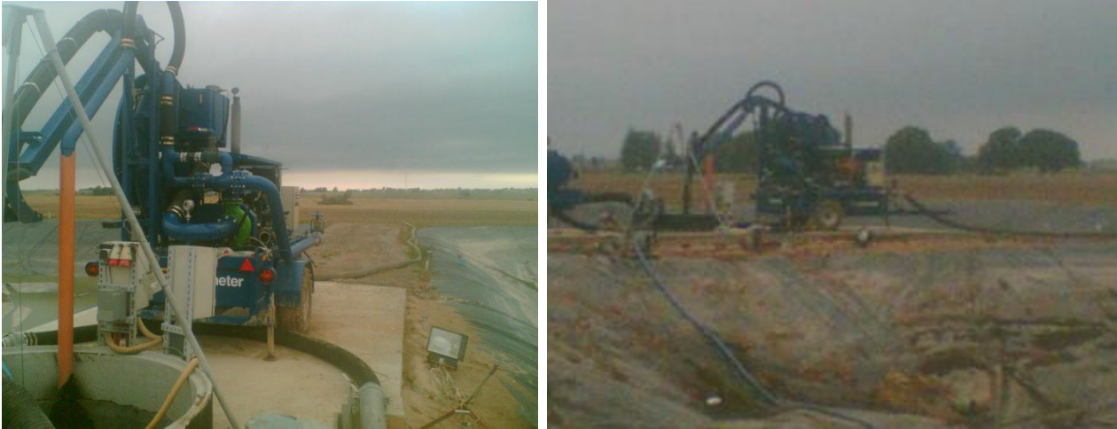
Figure 6.4.3. Mobile slurry pumping station used to pump slurry from the storage lagoons to the umbilical distributing spreader.
