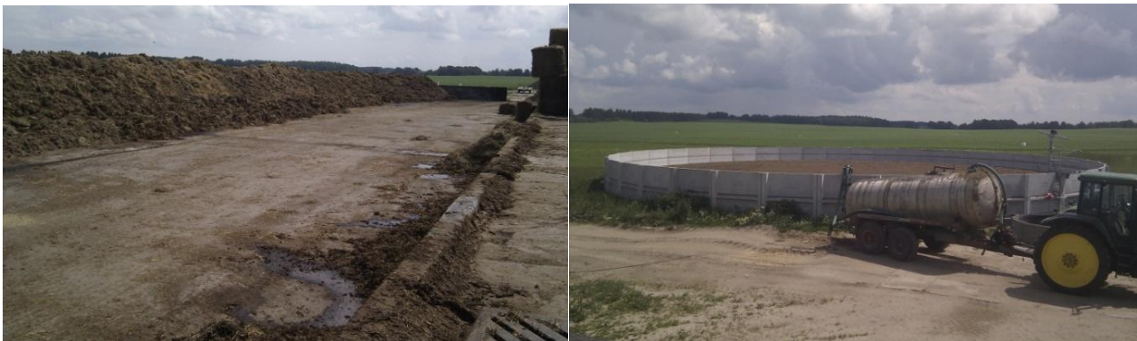
Figure 6.5.9. Outdoor concrete pad for solid manure (left) and concrete uncovered slurry tank (right).
