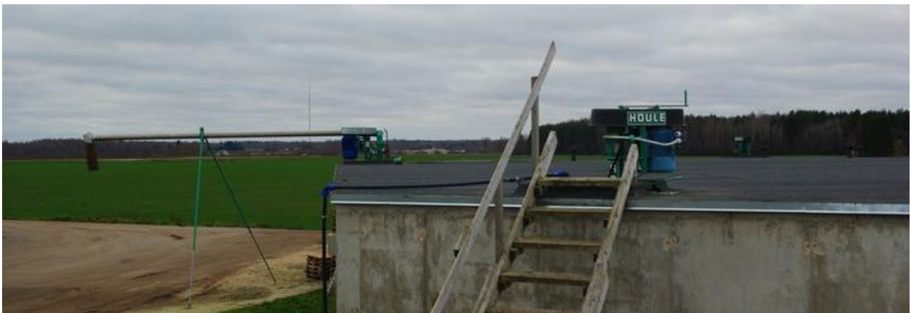
Figure 6.1.2. Picture of liquid manure storage tank (S) with stationary propeller mixers and unloading pipe.
