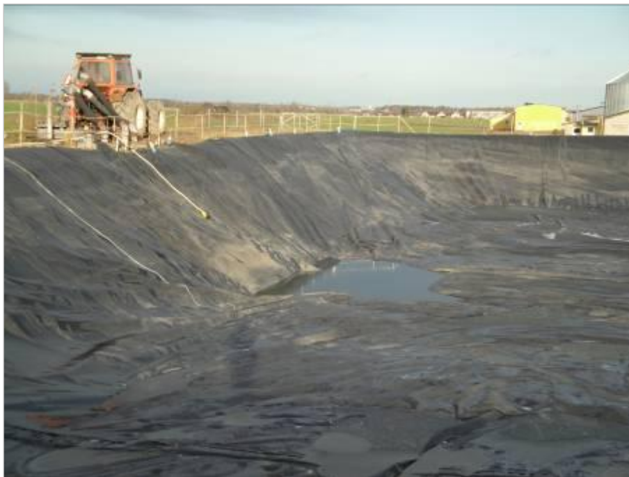
Figure 6.3.16. Covered storage pond for slurry.
