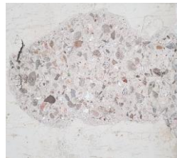
(b) Regional spalling
