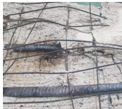
(c) Delamination at anchor (unbonded)
