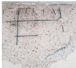
(a) Delamination at anchor (bonded)
