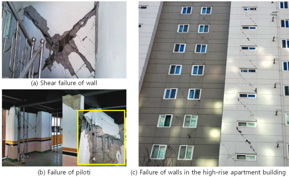
Fig. 1-1 Structural damages by Pohang earthquake
