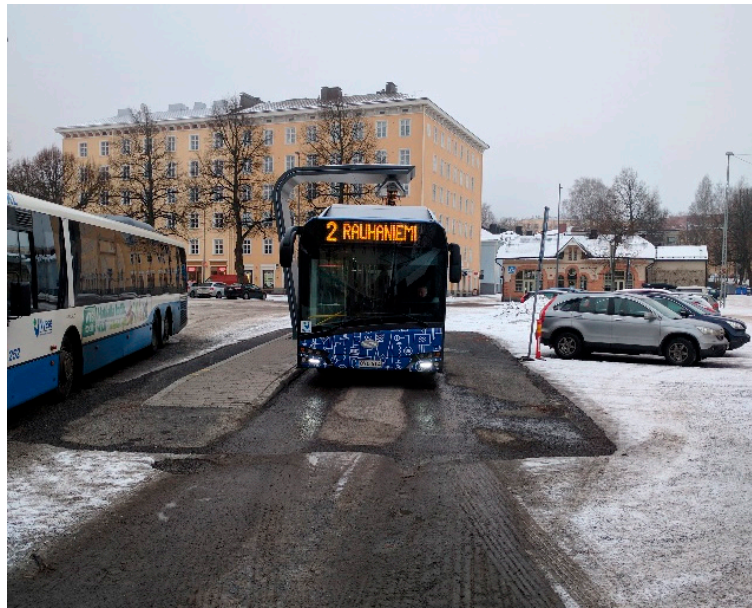
Figure 12. Heated foundation for the charging point to remove snow build-up on driving tracks.
