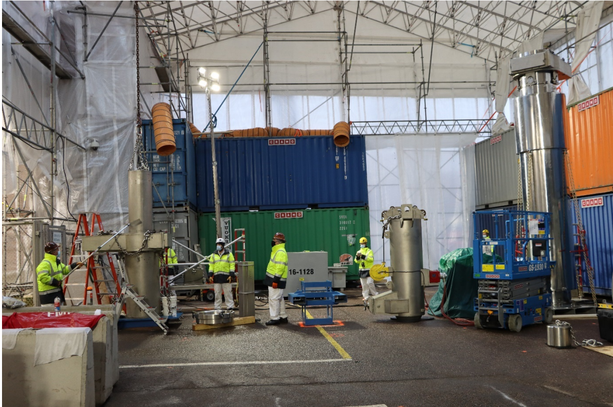
Figure 1. Site arrangements during fuel loading operations. On the left the transfer station of the Intermediate Transfer System (ITS). Here the inner shield with the loaded basket is lowered into the outer shield of the transfer station. In the middle the dry transfer system (DTS) and on the right the NAC-LWT cask. When the DTS is on top of the NAC-LWT for lowering the basket into the cask the total height of the system is 8 meters.
