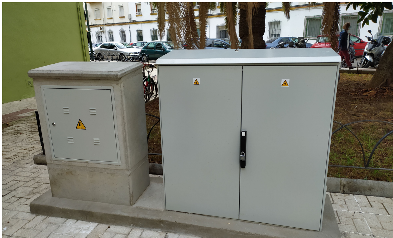
FIGURE 4. D-STATCOM prototype installed in a residential neighborhood in the city of Malaga. The power converter is installed in the cabinet on the right side, while the enclosure on the left side contains the shunt connection of the prototype to the grid, protection elements and measurements of the line downstream of the device.
