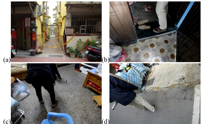
Fig. 4 (a) Damaged wall beside the front porch of a residence, (b) building subsidence caused by soil liquefaction, (c) formation of ridges on the floor of the house, and (d) cracks on the surface of the road and sandblast on the ground
