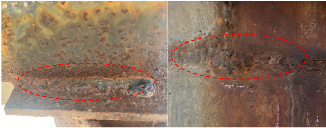
Fig. 1 Examples on corrosion at butt-welds and transverse attachment
