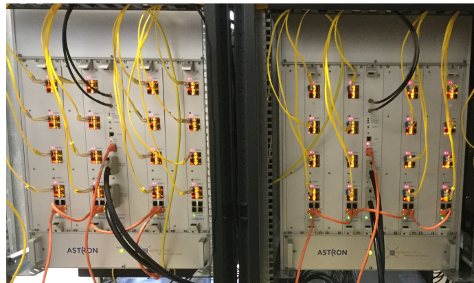
Fig. 22. Photo of two UniRacks in a telescope cabin (UniBoard side of the rack).
