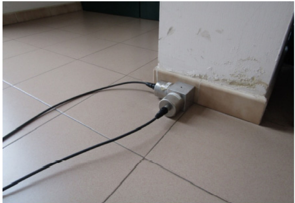
Figure 8. View of the sensors installed in one of the monitored points.
